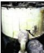
Asbestos lagging on an old tank
