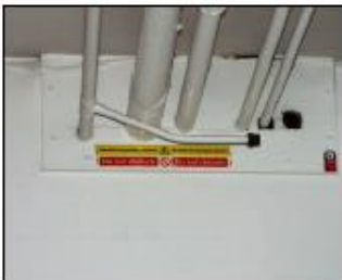
Don't assume there will always be warning signs. There could be undiscovered asbestos in buildings you work on.
