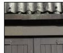
There could be sprayed limpet under this asbestos cement (AC) sheeting
